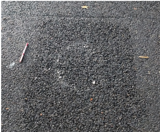
Figure 3 Permeable asphalt, Abbotsford St, North Melbourne
